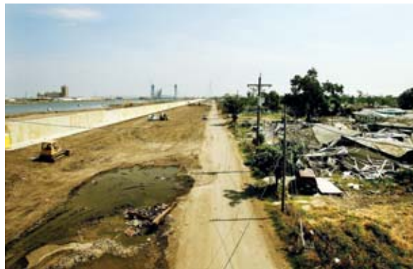
NEW FLOODWALL stands along the Industrial Canal, where a huge breach inundated the Lower Ninth Ward.
