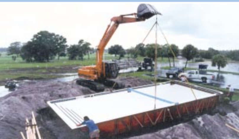
2 Place the Trident Fiberglass Pool into the excavation, run the plumbing and backfill the pool.
