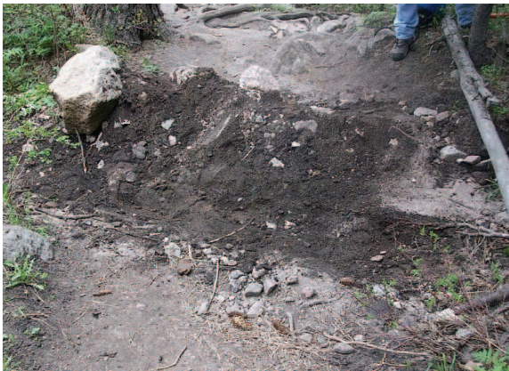
The side stream bed (darker color, right to left) is deeper, and a small wall built to prevent water from the side stream from flowing down the trail.
