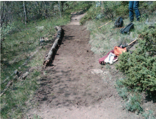
Berm removed from the downhill side of the trail and put into the trail tread to stop trail erosion in a gully; the tree trunk defines the edge of the trail so that users won't wander off the side of the trail tread
