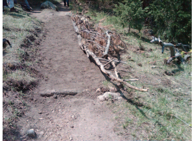
Another section of berm removal; the tree trunks and branches define the edge of the trail so that users won't wander off the side of the trail tread. A check dam (the log across the trail) holds the downhill end of the repaired trail tread in place as the trail starts more sharply downhill.
