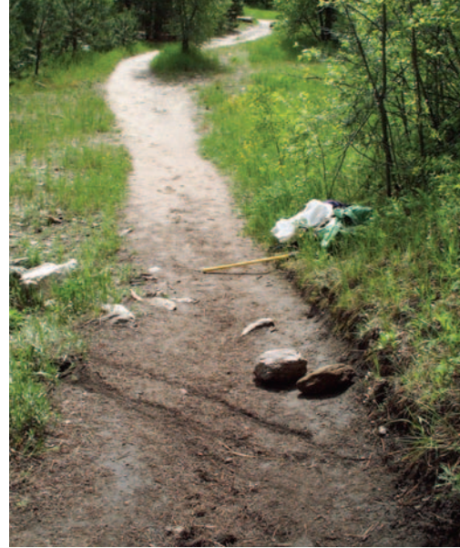
Before we put in the water bar, water was starting to erode the trail tread.
