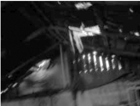
Ceiling of Noelvis's house
