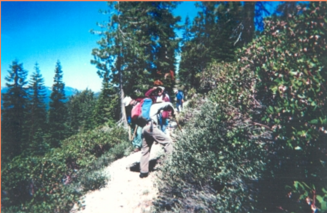
Photo by: John Lyons * Work crew on PCT section "P" between Gumboot Lake and Soapstone Lake.
